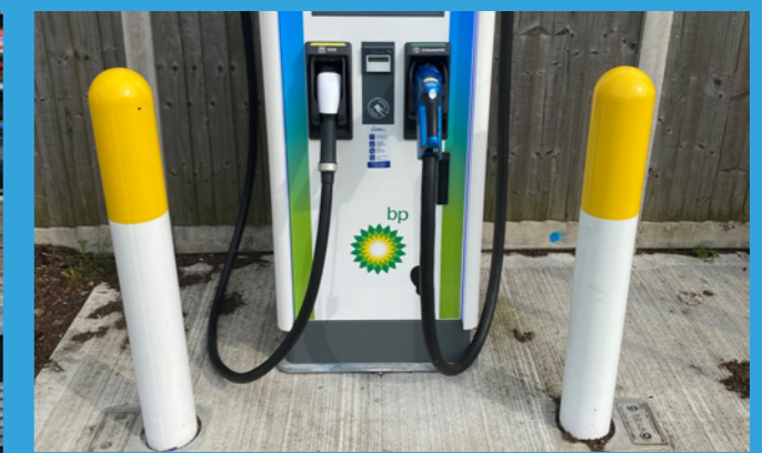
A barrier around a public rapid chargepoint
