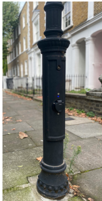
◀ A lamppost charger on a residential street.
